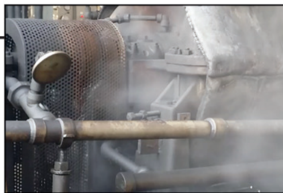
Steam leakage on process steam turbines increases steam costs and leads to lower efficiency and steam turbine performance.
